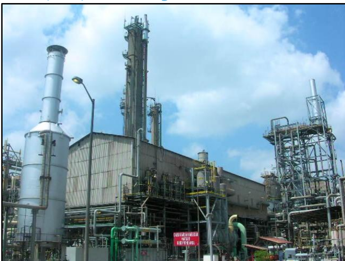
Figure 1. Ammonia Plant 1A of PT Petrokimia Gresik
