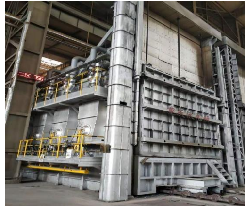
Regenerative Natural Gas Furnace after Retrofitting
