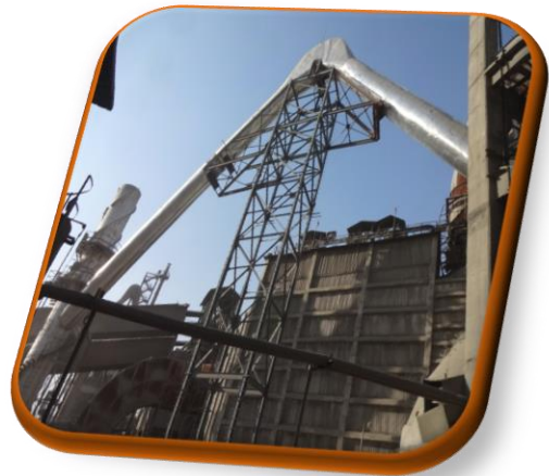
HOT-AIR RECIRCULATION DUCT
