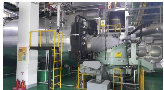
Fig. Wood pellet boiler of Laundry Factory
