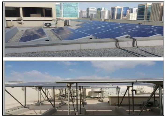
Photo No. (4): Solar System (PVT System) in ADM HQ & SCADIA Building
