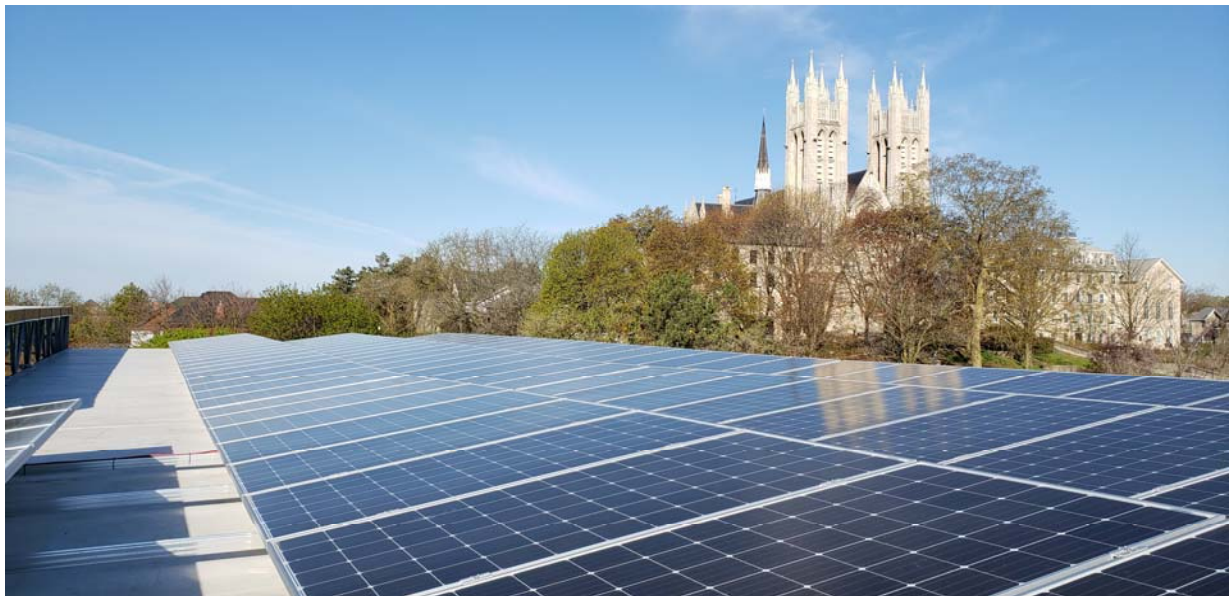
156kW Rooftop Solar PV System at one of the City-owned facilities
